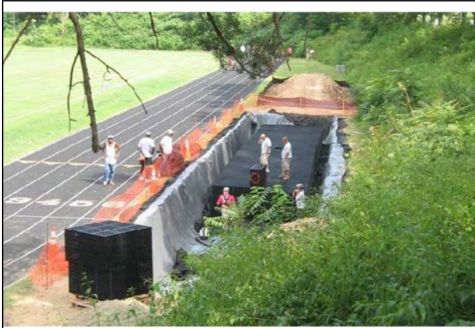
CHS Rainwater Harvesting – After (40,000 gallon system)
