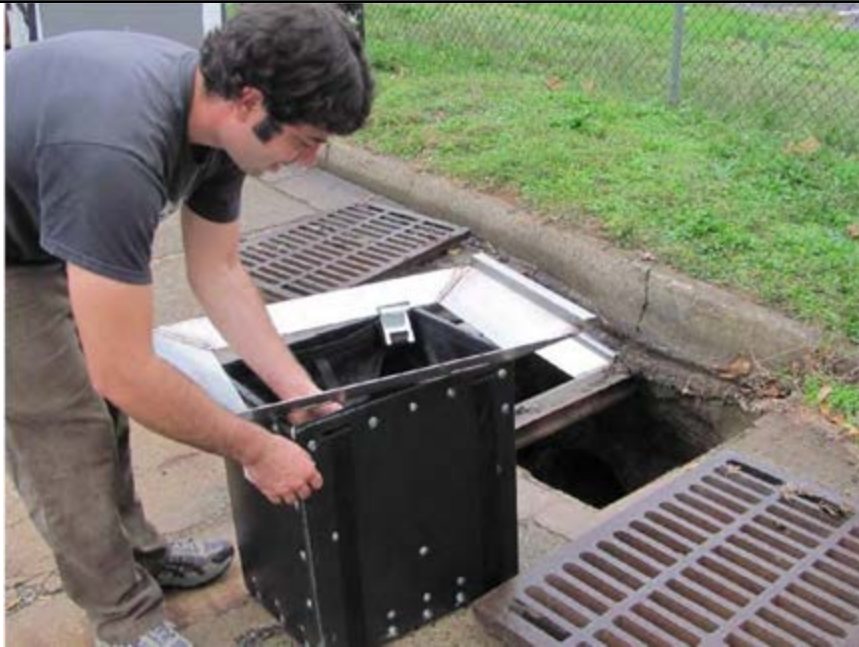
City Public Works Yard – Catch Basin Filter Inserts
